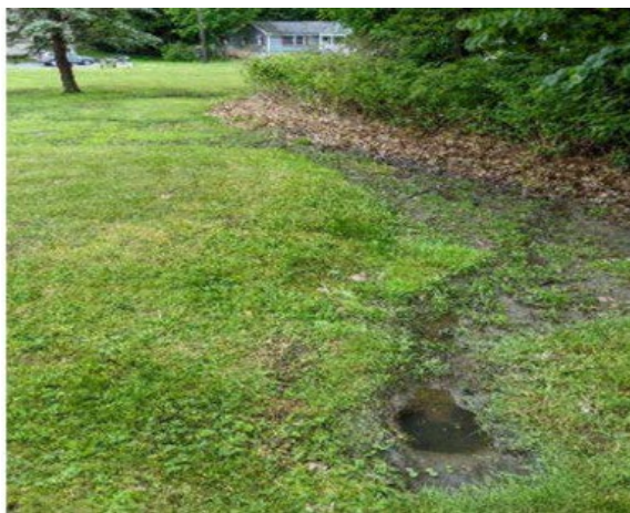
Fig. 3: The outlet of the Dept. drainpipe is submerged and drains to a yard with no outlet. The outlet should be daylighted and treated with a BMP (Site B). Source: UNH Stormwater Center
