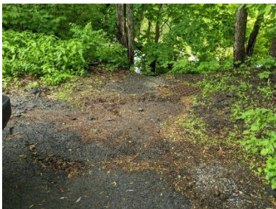
Fig. 1: End of road runoff avoids high catch basin and drains to paved swale left of basin. Source: UNH Stormwater Center
