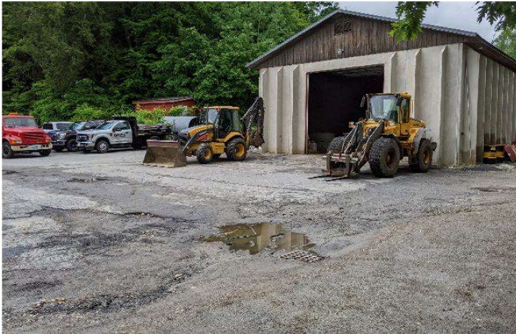
Fig. 1: The main catch basin for the Dept. drains half the garage, the lot, and the salt shed. It tends to back up during storms (Site A) Source: UNH Stormwater Center
