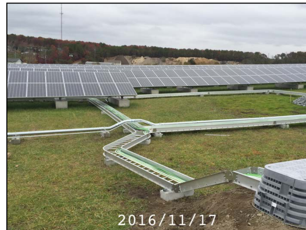
Use of above-grade cable tray collection system
