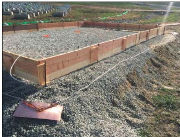
Use of Pad-mounted inverters
