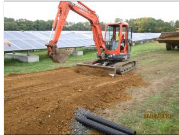
Improvement/creation of access roads to allow access to active gas collection systems
