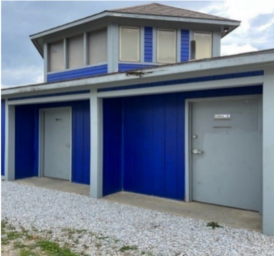
No ADA Signage for Restrooms
