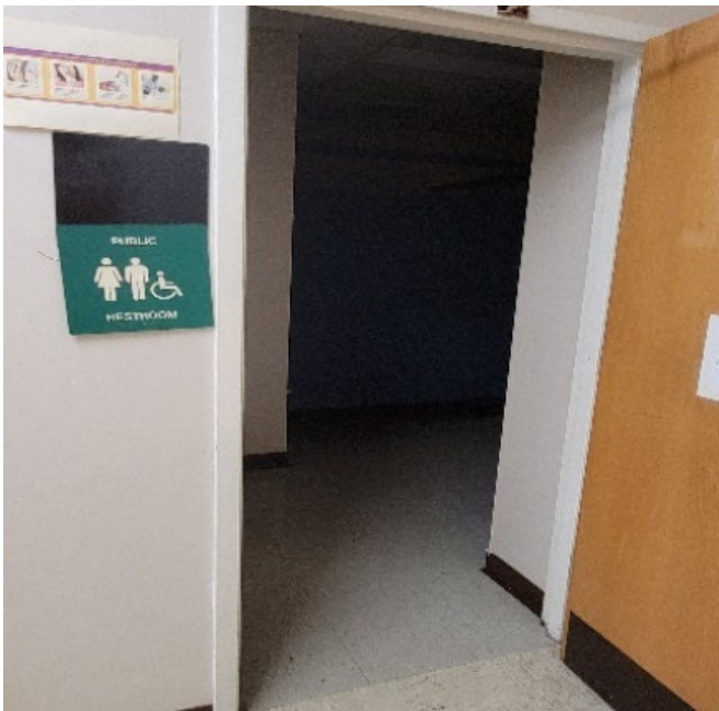
Signage required in Braille & 60" above floor Additional modifications needed to ADA dispenser heights, signage, and entry.
