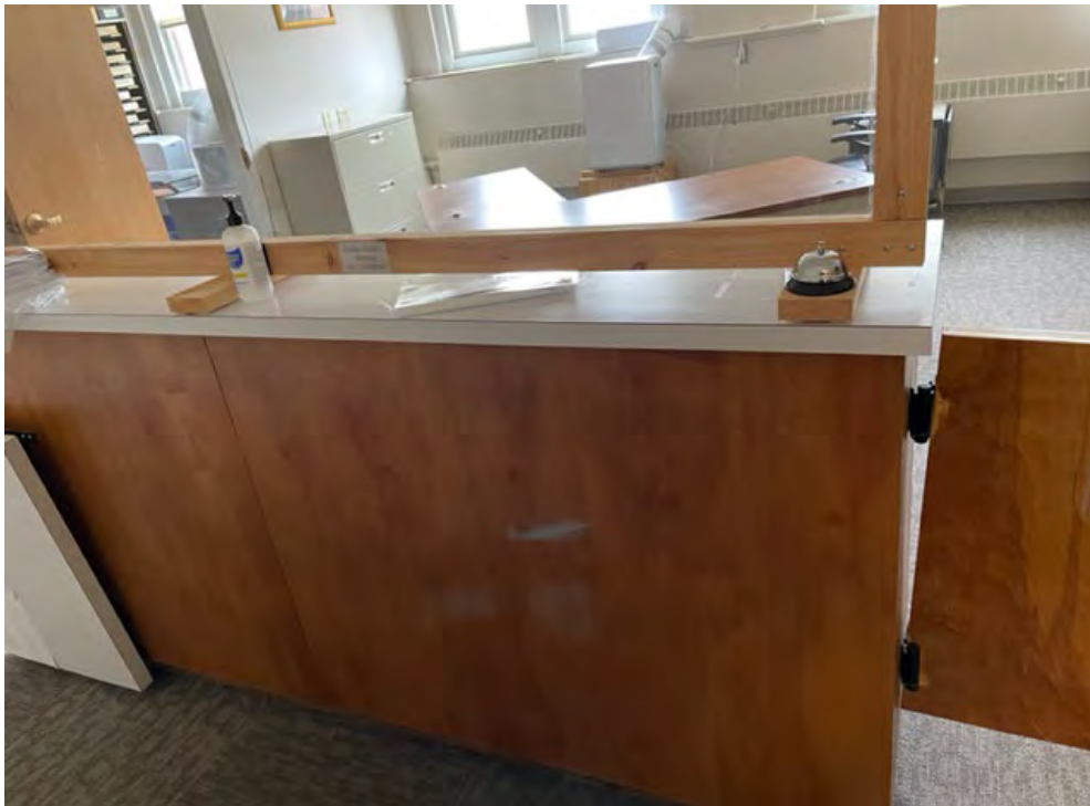
No wheelchair accessibility - Service Counters require section at accessible height
