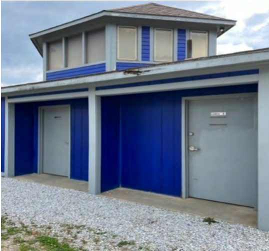
No ADA Signage for Restrooms
