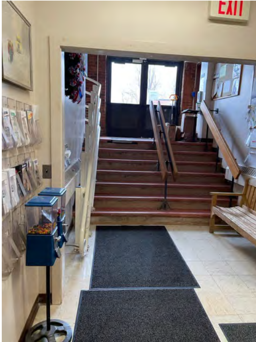
Inside entry of the Police Station; no elevator, ramp or lift
